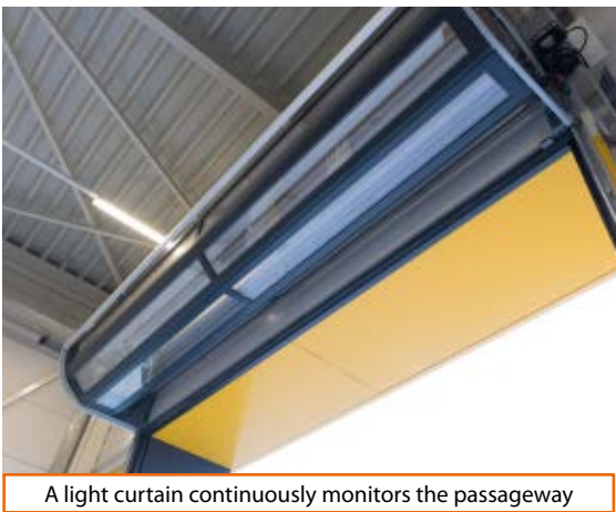
A light curtain continuously monitors the passageway
